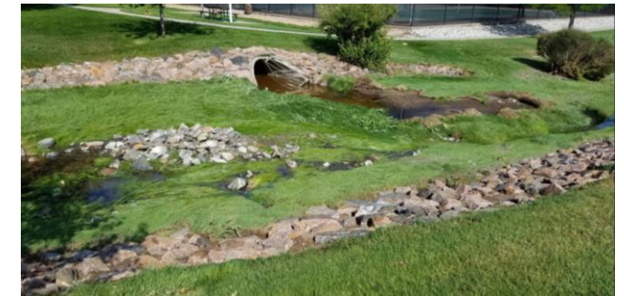
Fox Hill Park Tributary overtopped East Kettle Drive and eroded turf along the drainageway
