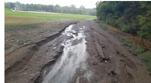
Homestead Farms Tributary escaped the left bank eroding the pedestrian trail near Homestead Elementary
